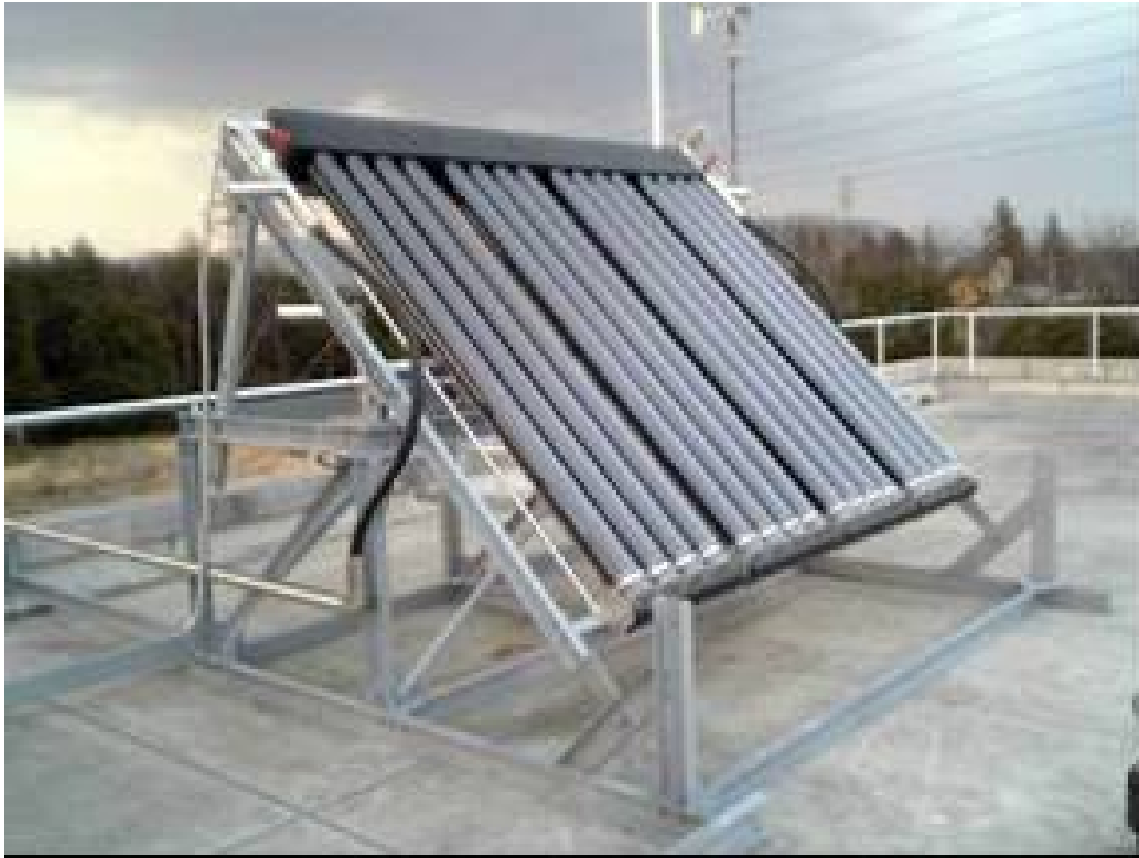
Solar Hot Water System
