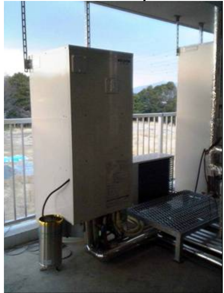
CO 2 heat pump Hot Water System
