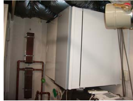
ventilation unit with a heat recovery element
