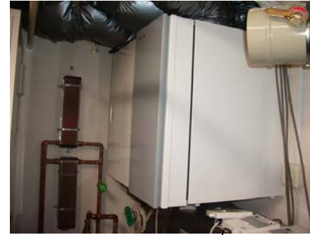
ventilation unit with a heat recovery element
