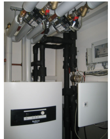
The heat pump and the measurement equipment
